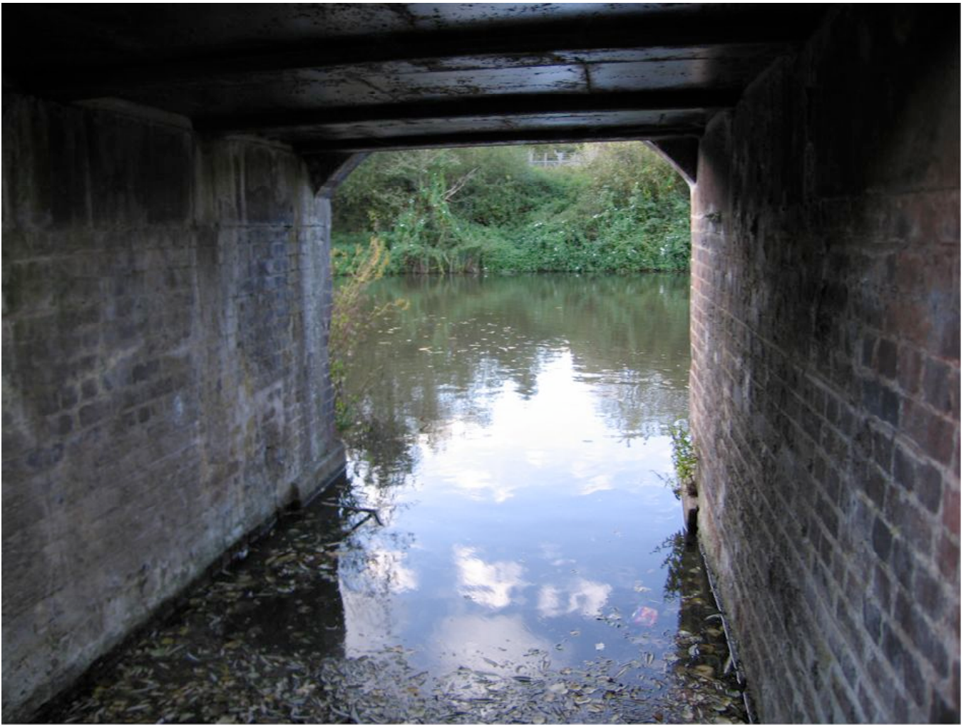
The old entrance to the wharf under the restored over bridge. Viewed towards the canal
